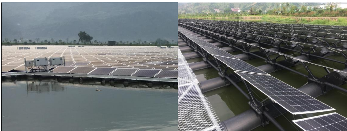
Figure 4: Zhejiang Jiande Floating PV plant utilises SUN2000-50KTL inverters
