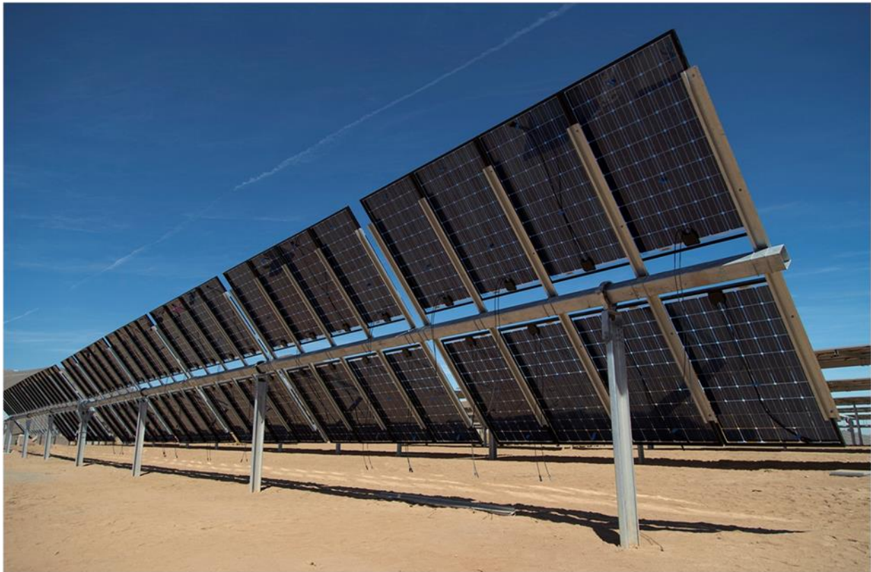
Figure 1: Bifacial PV modules installed on a tracker 1
